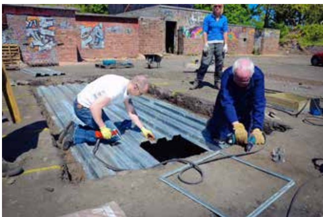
On a sunny day in May 2014 we capped the SOC sewerage pit. This is three of our volunteers riveting the troughing together before we fitted high-tensile steel reinforcement mesh and poured the concrete
